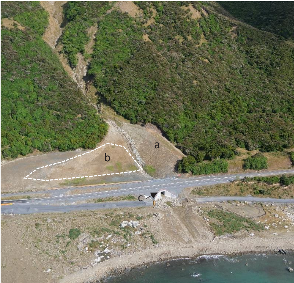
FIGURE 46: Open Control Structures at Jacob’s Ladder (a) lateral berm (b) depositional basin (c) large dimension culvert under the transport corridor for conveyance of residual flow. Photo courtesy NCTIR.
