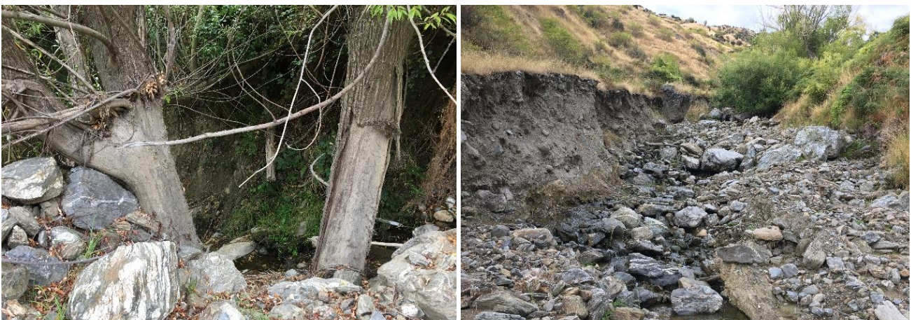
FIGURE 13: Left - Impact scars along vegetation above current channel level; Right - Active bank erosion in colluvium and partial deposition of bouldery debris within the main channel.
