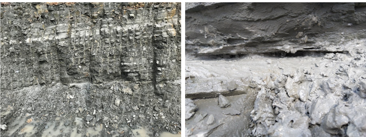
FIGURE 17: 10 mm wide parallel bedded clay seam comprising highly saturated light grey clay in East Coast Bays Formation rock excavation. Moisture content of the clay seam was measured at 62.2%. Ring shear tests carried out on the clay infill recorded effective residual friction angles, \phi_r^* , of 10° and 19° ( c_r^* = 0 kPa).
