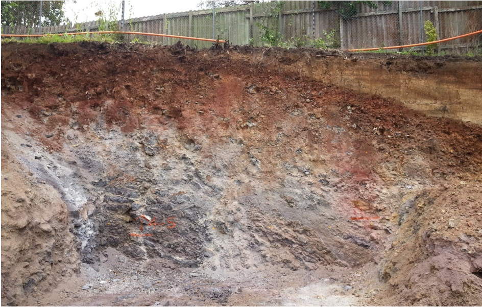
FIGURE 32: Sub-vertical temporary cut slope in partly welded scoria overlain by ash and tuff in Auckland Volcanic Field prior to anchor installation. Performance of cut slopes in this geology is governed by blockiness, soil layers of different permeability, and groundwater levels.
