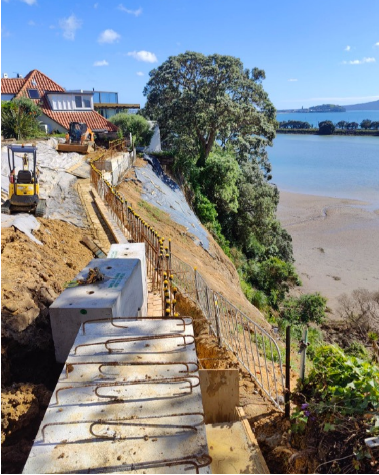
FIGURE 36: Figure 36: Construction of a palisade wall with concrete capping beam in East Coast Bays Formation in a coastal cliff setting.
