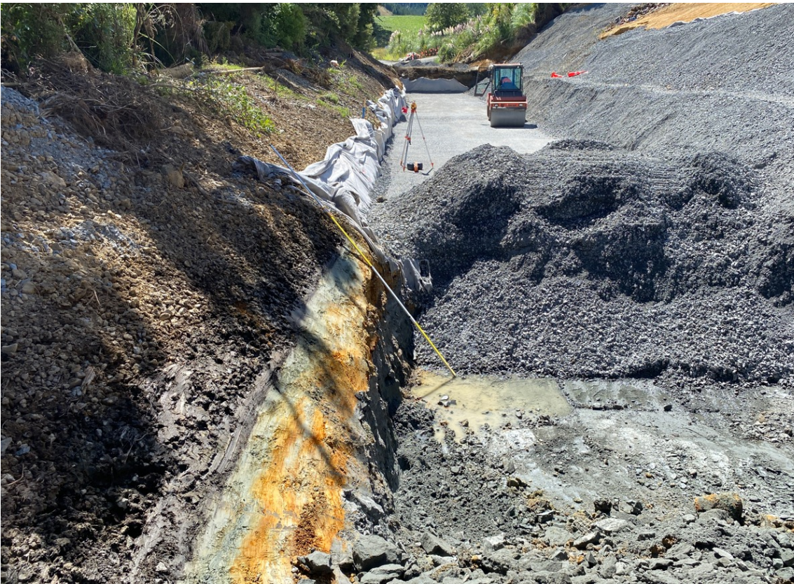
FIGURE 35: Hardfill being placed and compacted in a shear key excavation at the toe of a creeping translational block slide in Pakiri Formation.
