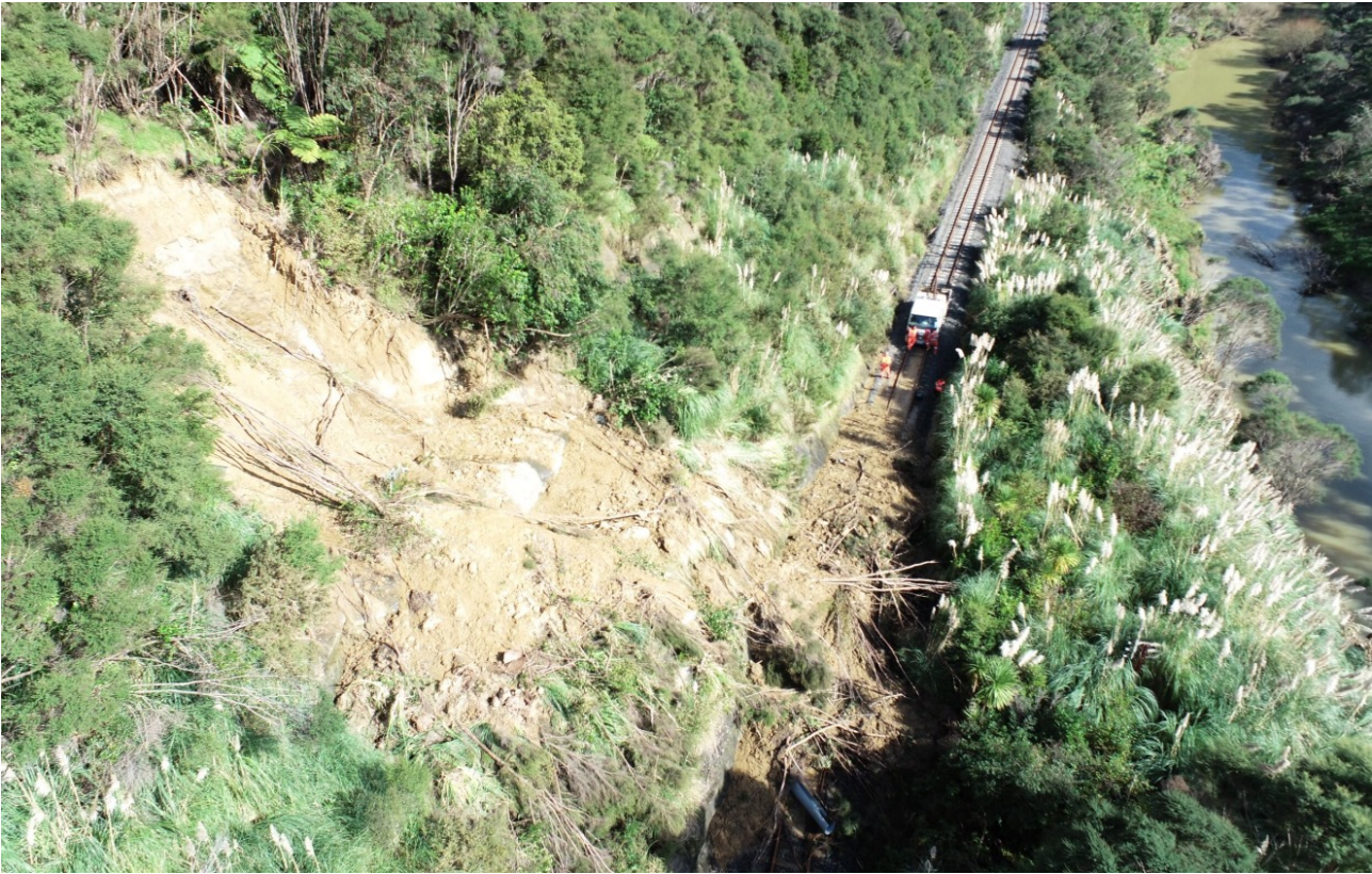
FIGURE 23: Debris avalanche in Pakiri Formation residual soil overlying rock. Saturated soil and entrained vegetation flowed over the rock shelf to inundate the railway line.
