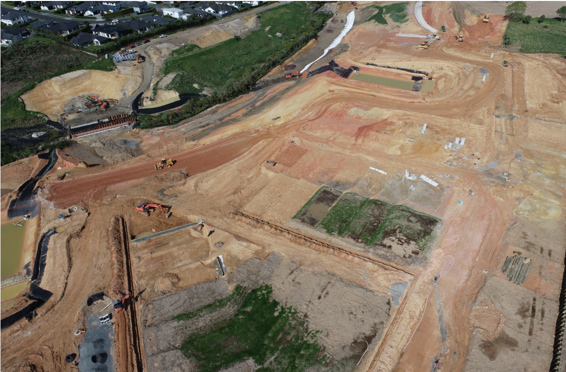
FIGURE 33: A conventional bulk earthworks site for residential subdivision in Auckland. A specialist earthworks contractor is recommended to manage a site of this nature, where installation of critical geotechnical stabilisation measures governs the civil earthworks design.
