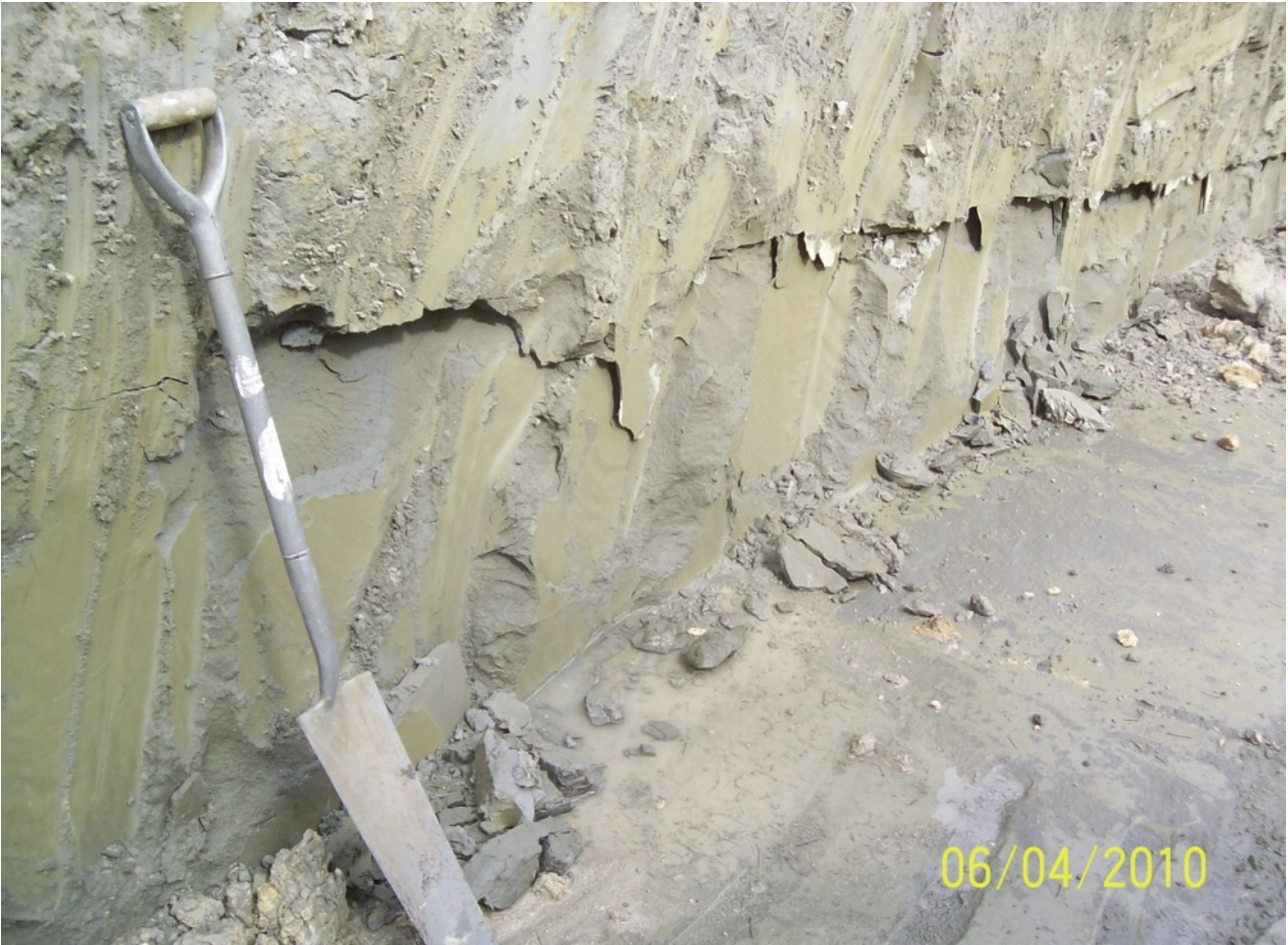
FIGURE 16: Parallel bedded clay seam in residually weathered East Coast Bays Formation sliding into a shear key excavation at a rate of approximately 20 mm/day.
