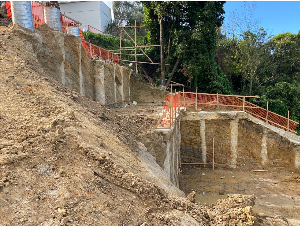
FIGURE 37: Tiered palisade walls to support building development on a steep slope in East Coast Bays Formation , with excavation after construction to support building development.
