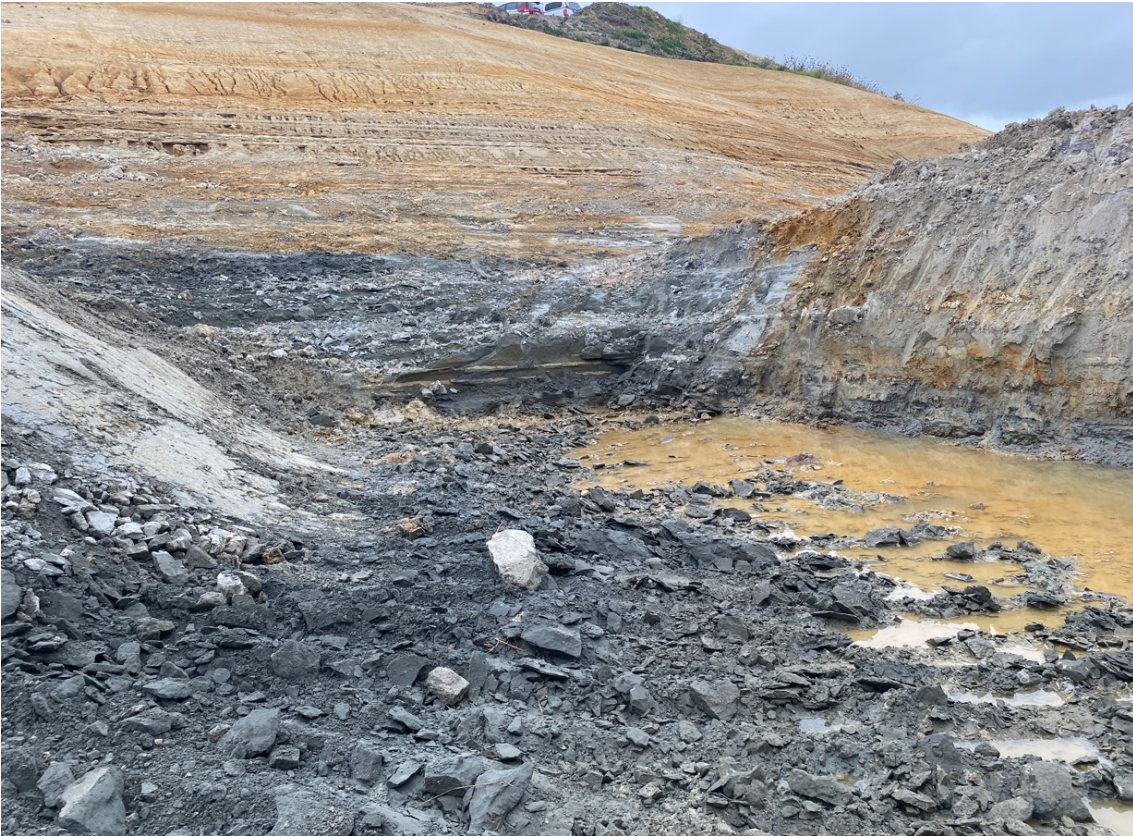
FIGURE 34: Shear key excavation in deeply weathered East Coast Bays Formation residual soil and very weak rock. Temporary stability of the excavation is managed by sequenced excavation and backfill placement over short sections. Fill wedge at left, intact ground yet to be excavated at right.
