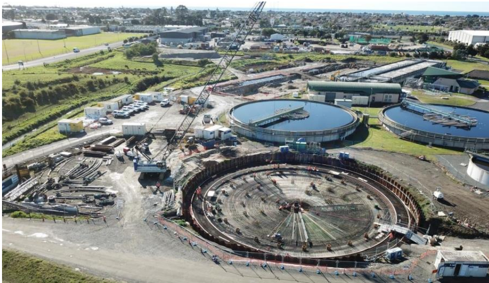
Figure 6. The new clarifier (at the bottom of the image) with piling completed
