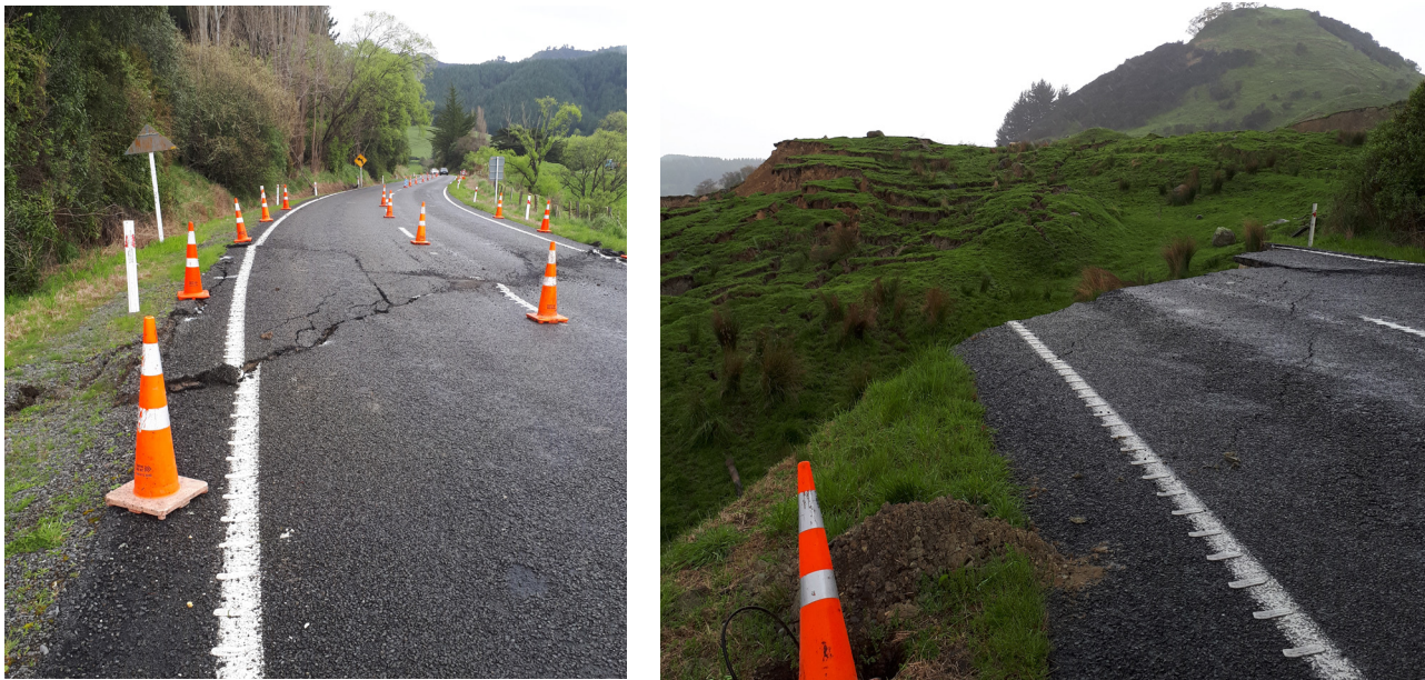
FIGURE 5: Surface cracking mapped prior to failure (left), and the lateral scarp of the landslide at the same location of the mapped cracks following failure (right).
